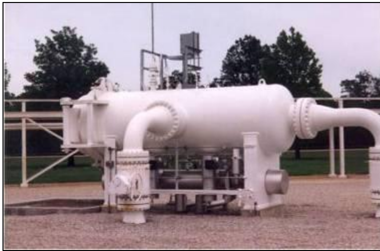
Natural Gas Filter-Separator
