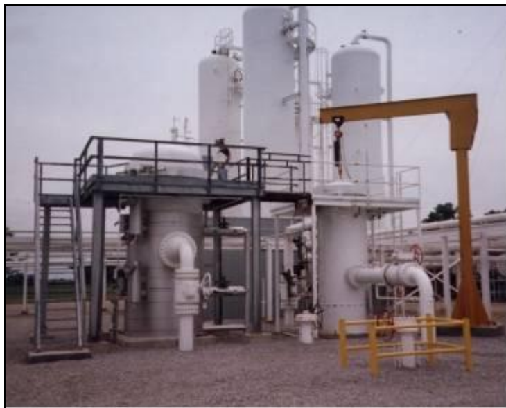
Inlet Gas Coalescers, note towers in background
