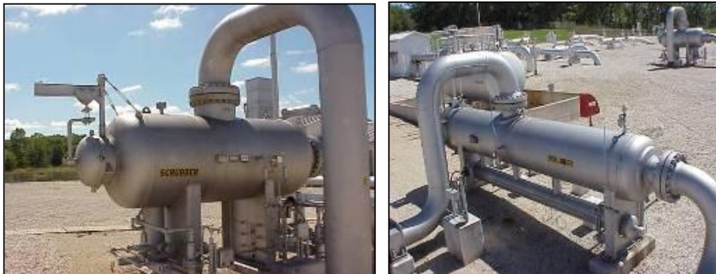
Natural Gas Filters (Note Vertical or Horizontal Liquid Sumps below Vessels)
